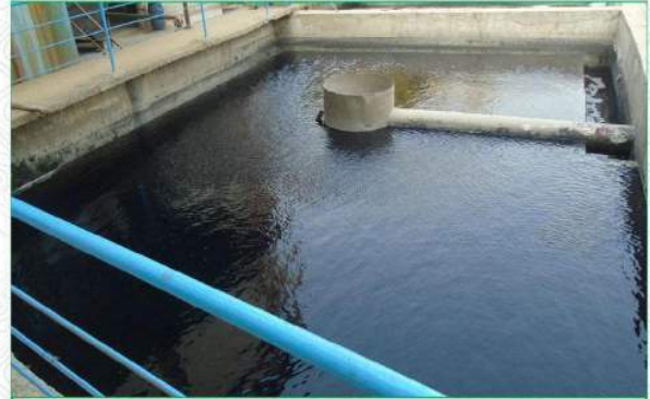
10) Double Chamber Clarifier
