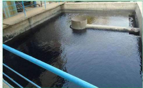
10) Double Chamber Clarifier
