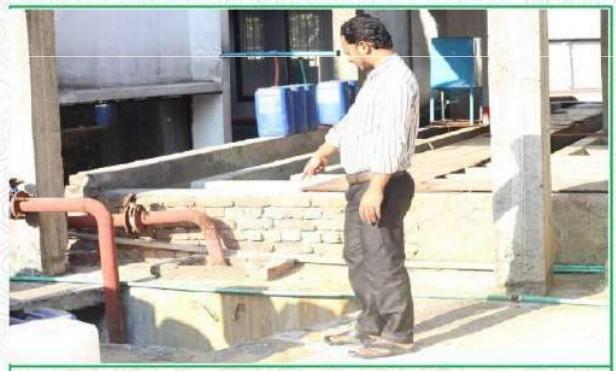
4) An aerobic Digester 1
