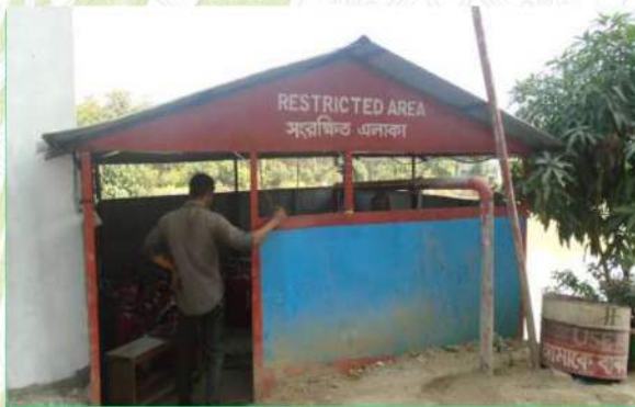
Water pump for fire control
