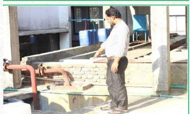
4) An aerobic Digester 1
