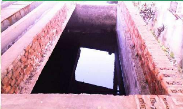
5) An aerobic Digester 2
