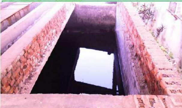
5) An aerobic Digester 2
