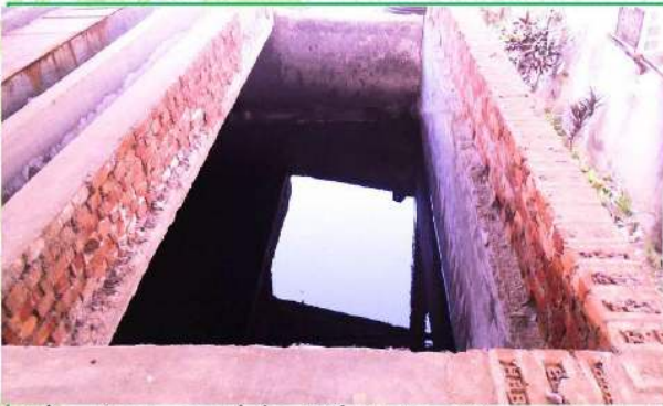
5) An aerobic Digester 2
