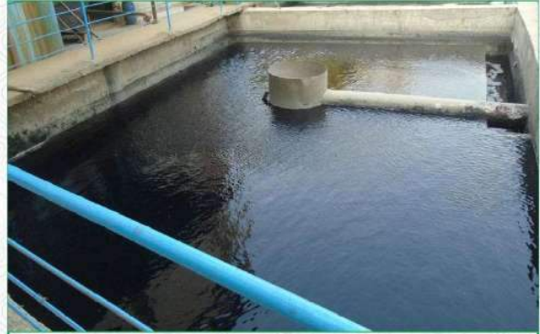
10) Double Chamber Clarifier
