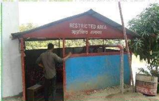
Water pump for fire control
